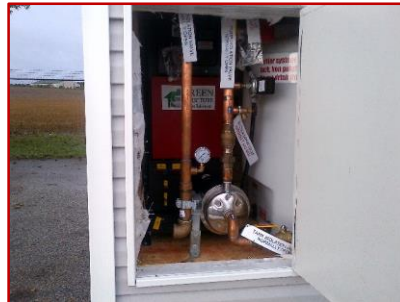
➤ Tank & Pump Interior
